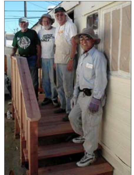
David McCreath, Rod Thorn and Bill Ribble on the porch and steps they built for a Western Trailer Park resident (the man in front is a volunteer from Fujitsu, which helped with both funds and volunteers)
